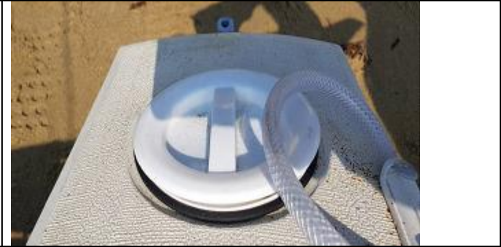
Cross threaded hatch cover will not seal
